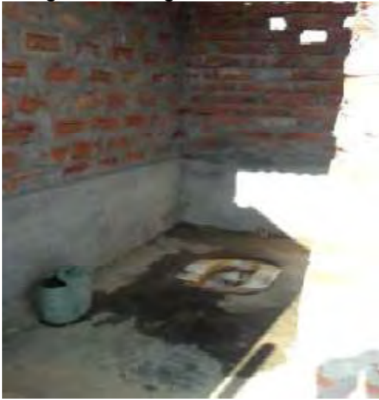
Toilet facility for workers
