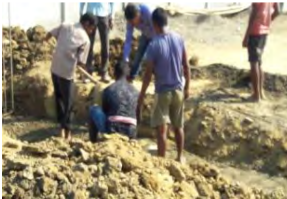
Boundary wall under construction. No use of PPEs by workers
