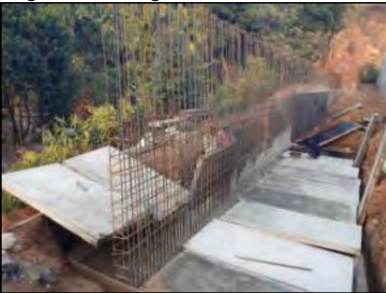
Shuttering works of Retaining wall (Extended Portion) at Gopal Nagar in Progress
