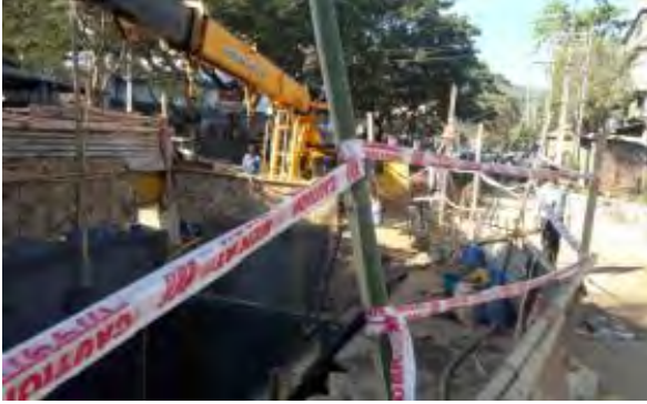
Permanent barricade arranged at pipe laying area of Barbari. Deep excavation noted
