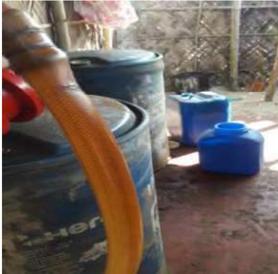
Fuel stored in separate storage but no oil tray noted below the fuel storage drum
