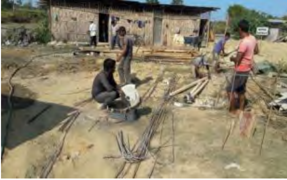
No use of PPEs by workers during rod cutting and bending
