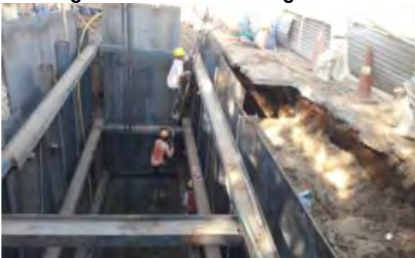
Partial use of PPEs by workers at Barbari site micro tunneling area
