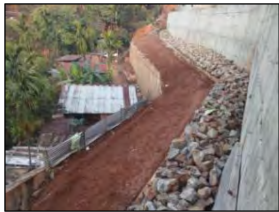
Preparation of Bed for Stone pitching behind Retaining wall at Gopal Nagar in Progress
