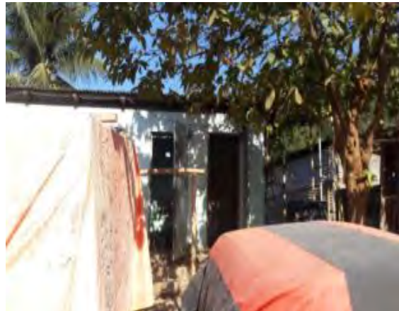
Toilet facility at Gopalnagar site adjacent to labour camp
