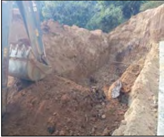
Excavation of Soil for Construction of Retaining wall at Kenduguri Reservoir site is in progress
