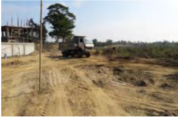
Dust suppression through water sprinkling done. Which needs to be continued as per requirement
