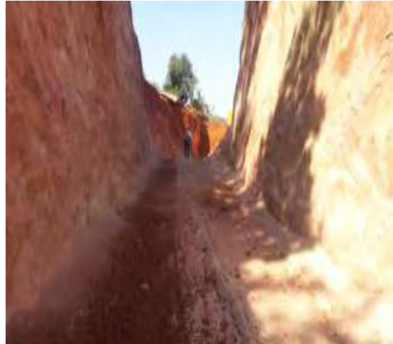
Earth cutting done for approach road at North Jyoti nagar reservoir site
